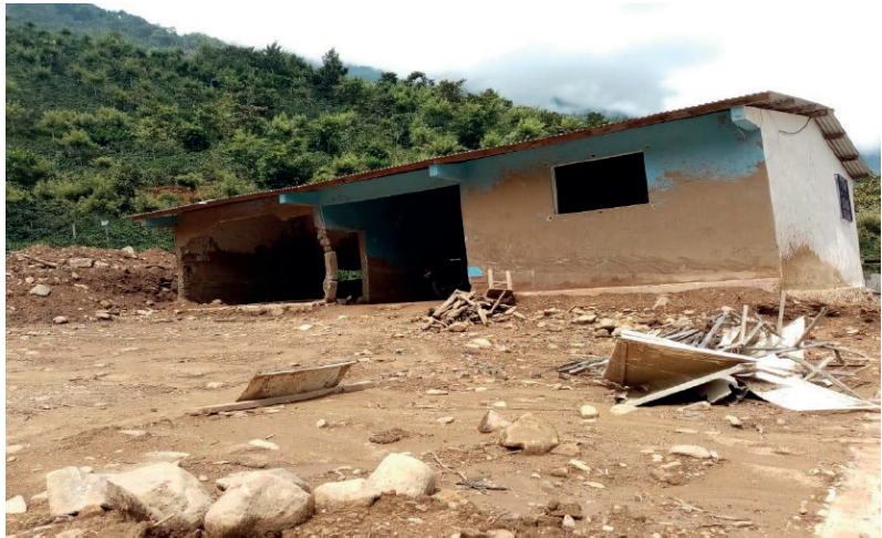
Devastated health centre in El Boquerón 2020
